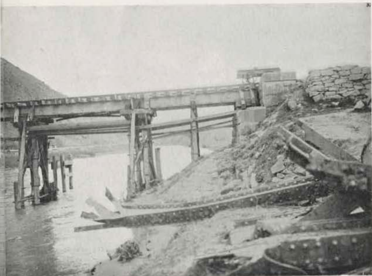
Line Belgrade-Nish-Vranje, 302 km. 550. Destroyed iron bridge of 54 metres opening over the Morava river at Grdelitsa and temporary repairs
